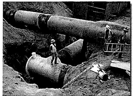
72-inch pipeline at SJWD WTP
