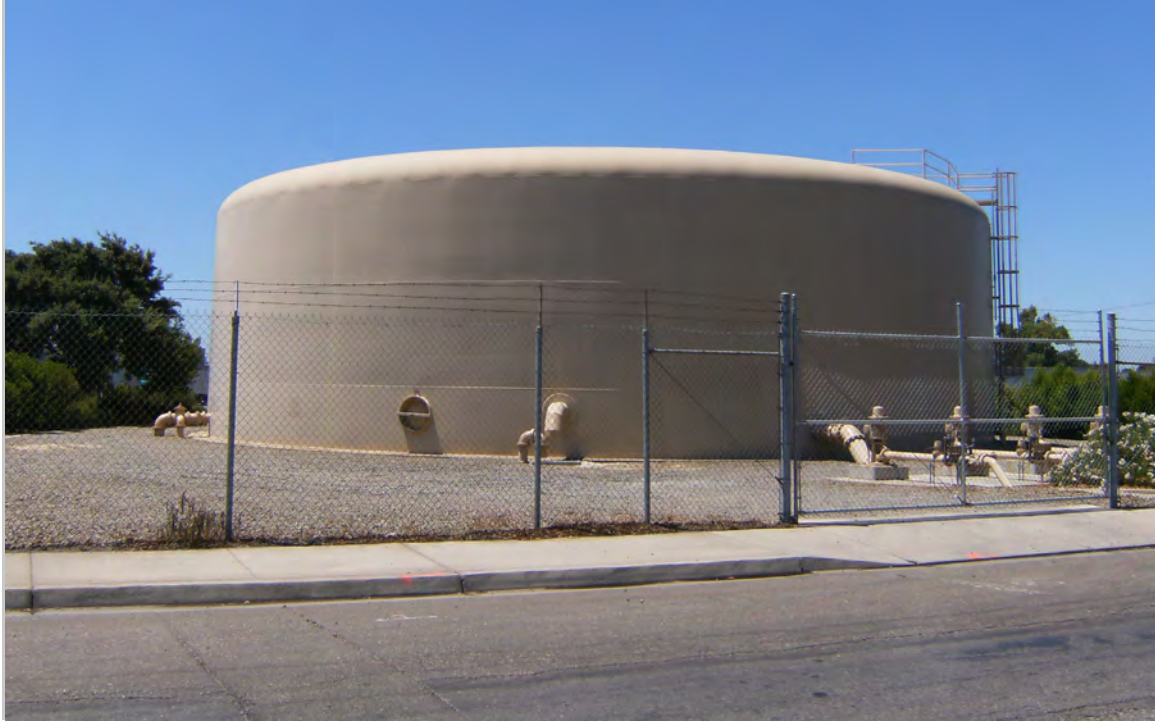
Photo 1. Water storage tank with booster pump stations.
