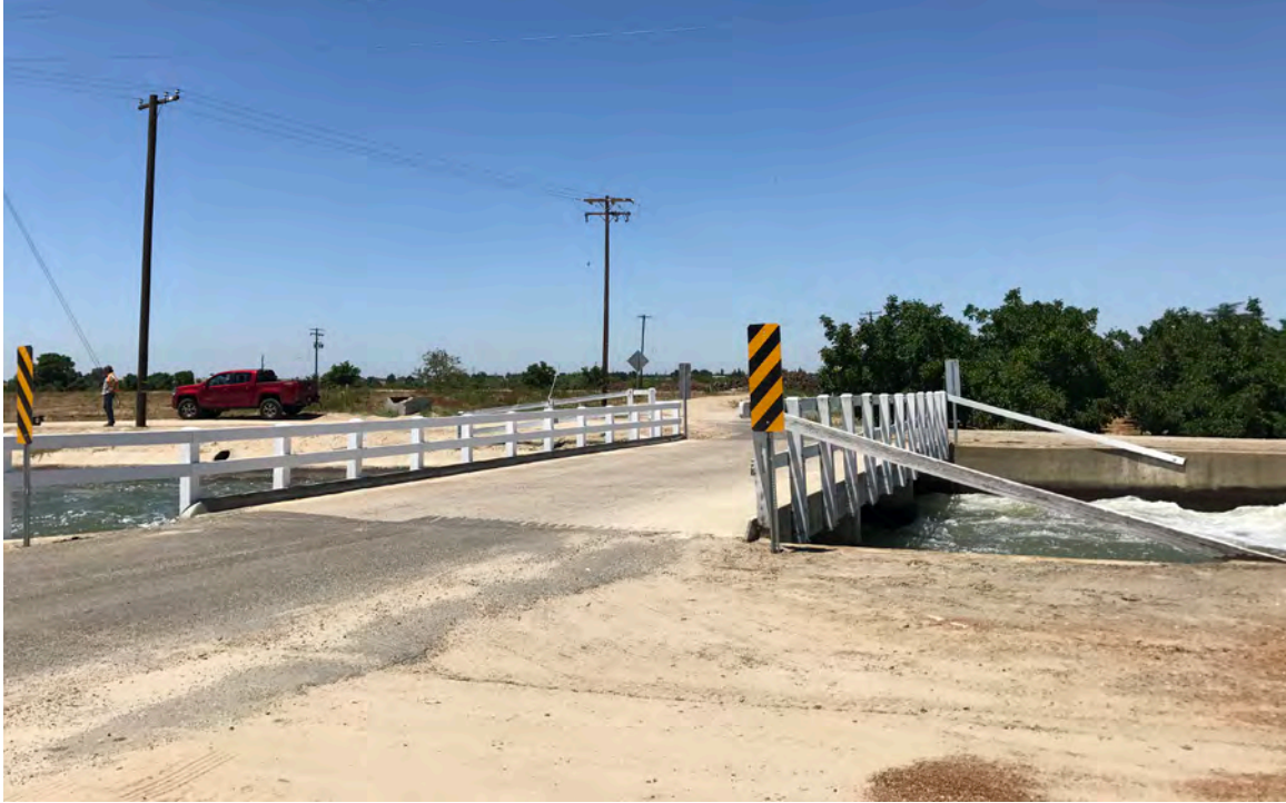
Photo 3. North facing view of the Aldrich Road crossing over the Ceres Main Canal. (June 2017)
